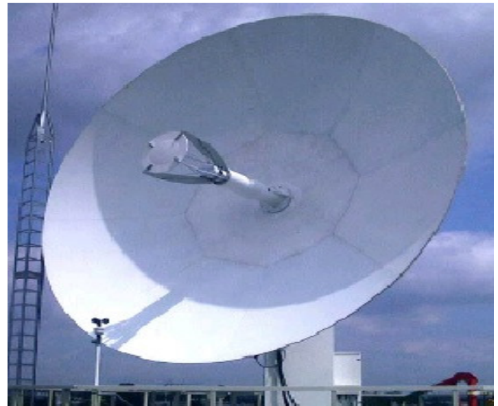
Fig. 9. X-band dish antenna at Murezeg station
