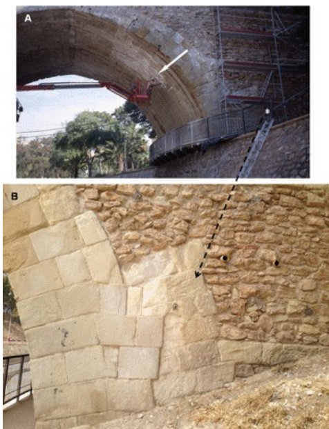
Fig. 2 South side of the bridge. A. Cleaning and sampling of salt vault efflorescence (arrow) (2005). Asterisk shows the preferred study area in this paper. B. View of sampled abutment of the bridge at 2008.
