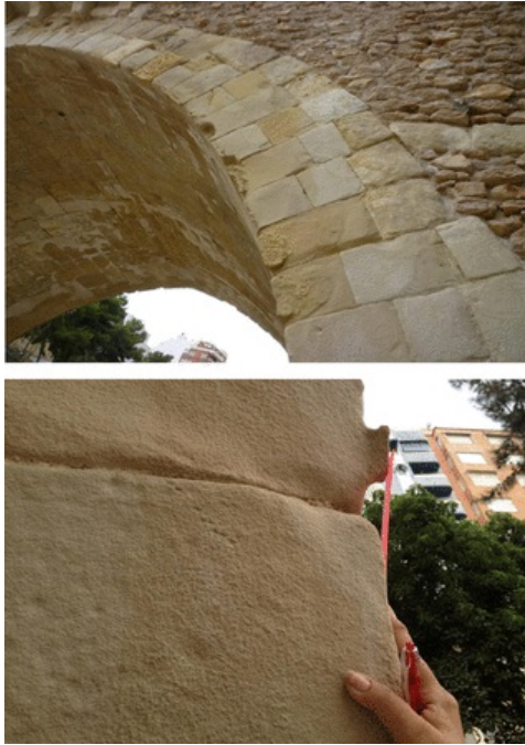
Fig. 5 Erosion on the corners of the south wall. July 2013.
