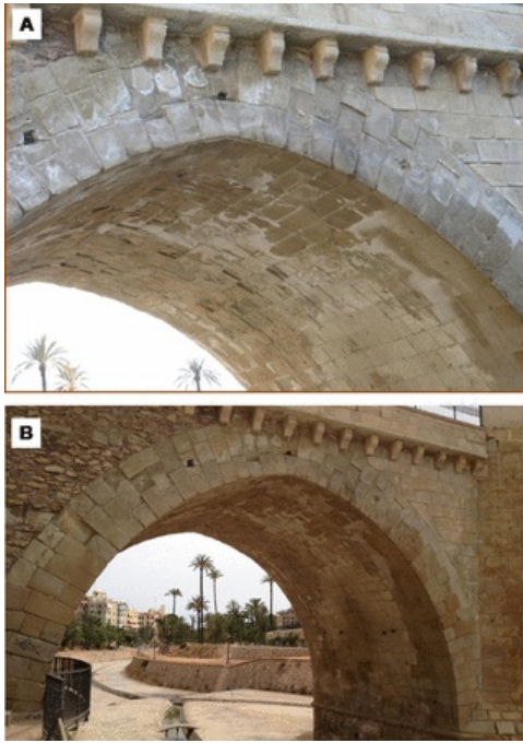
Fig. 3 Efflorescence on the N face of the arch and on the vault. A. At 2008, B. North face of the arch at 2013. Outer surface is free from salts, but flaking and contour scaling are evident.
