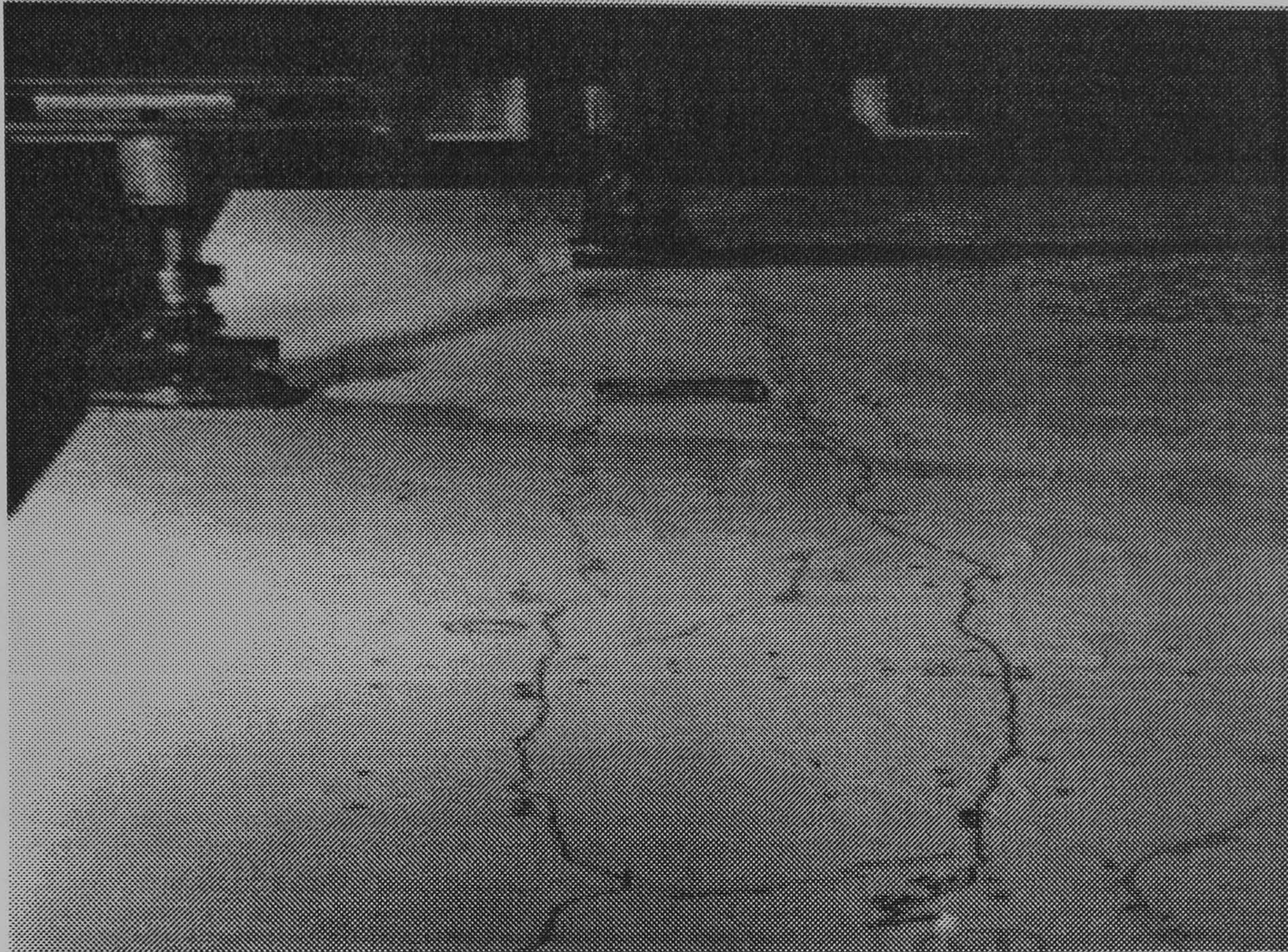
Figure 8.12: Crack pattern in test TR1P2
