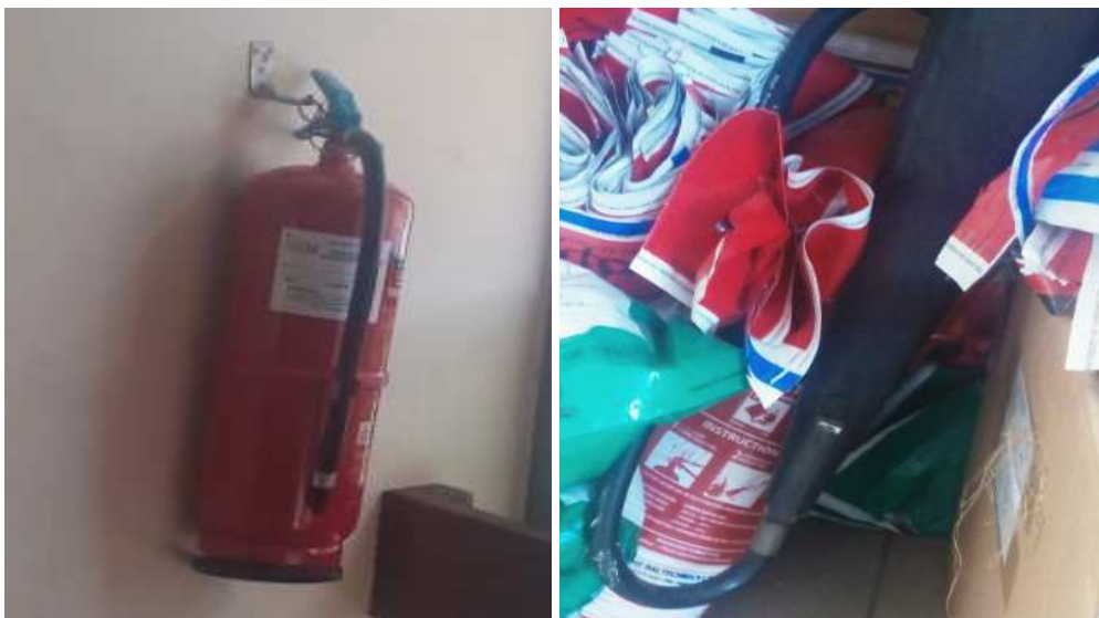
Figure 4.18: Fire Extinguishers in ODL Tower and Block C at OUT
