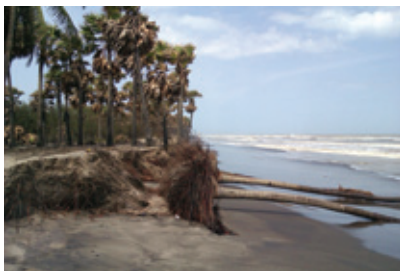
Coconut trees damaged by sea erosion at Peddamylavani Lanka
