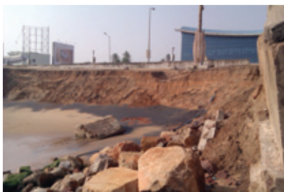
Sea erosion at Ramakrishna Beach
