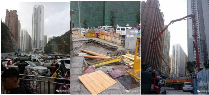
Messy onsite parking Poor safety management Dangerous construction operation
