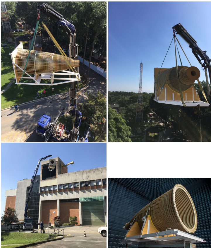
Fig. 8 Top left, top right and bottom left: Horn being suspended, with its cart, to the opening of the anechoic chamber of LIT test facility. Bottom right: The horn mounted inside the anechoic chamber.
