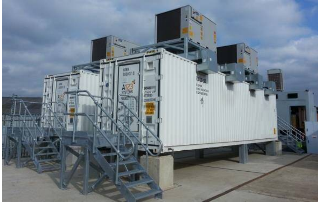
Figure 2.5. Element Power’s 12.5 MWh battery storage project, which secured one of the most remunerated contracts in last year’s EFR tender by National Grid [75].
