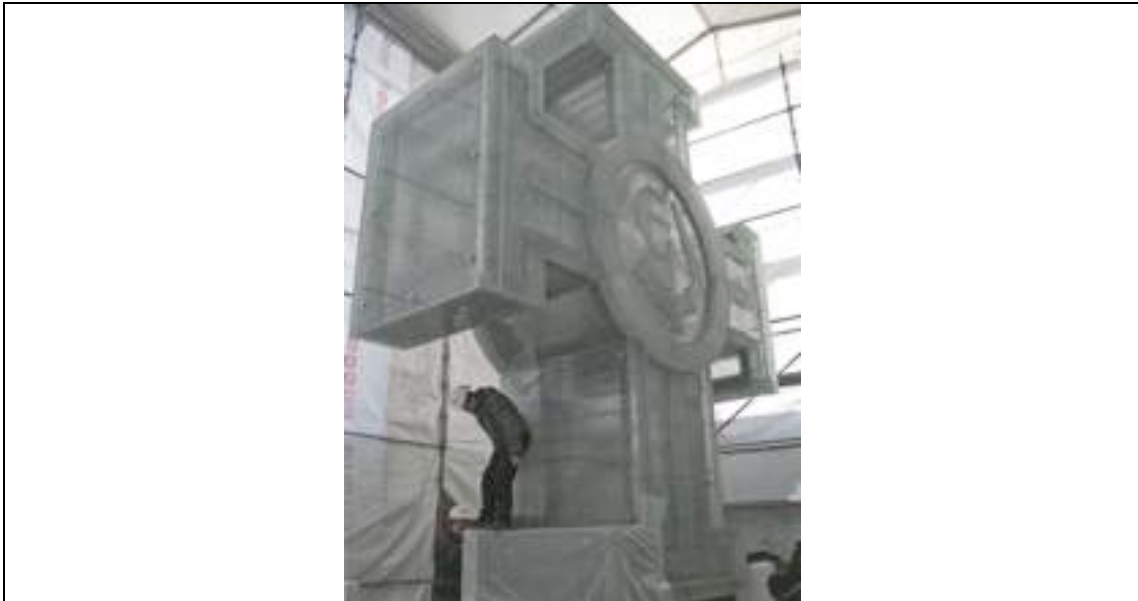
Fig. 21 – The Cross of Liberty at the top of the Victory Column during the constructions.
