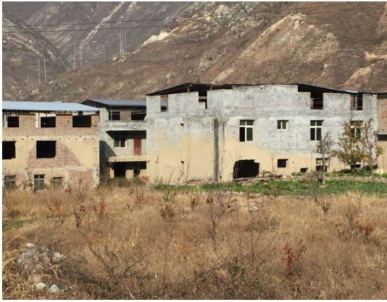
Figure 5: Flow-type slide damage on buildings in Qipan Gully
