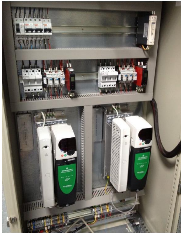
Fig 4.3 Inside view of cabinet containing Unidrives
