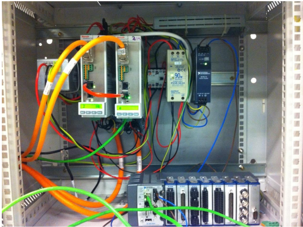
Figure 7.15: Motor drives and Compact RIO arranged in the drive cabinet.
