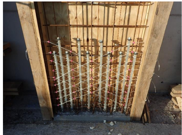
Figure 9: SMP and flow network arrangement fitted in Panel B
