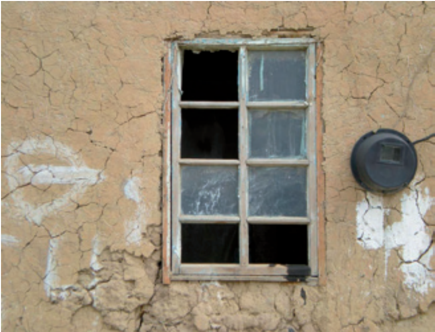
Picture 5. Insulation problems in informal settlements in Kyrgyzstan
