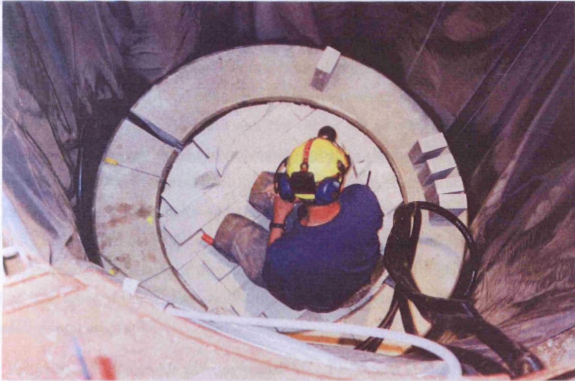
Figure 6.15. Installation of the bentonite bricks on the top of the canister (Johannesson et al. , 2004).
