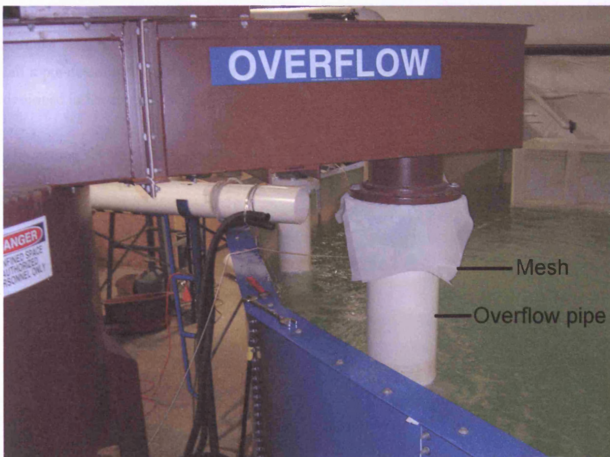
Figure 7-3. The placement of the mesh at the overflow in the 6' diameter Grit King ® .
