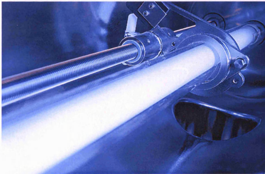
Figure 63:- Inside of a UV water treatment chamber.[60]
