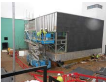
Sequence showing construction build-up of cement particle boards on steel SFS framing, taping to provide weathertight and airtight seal, insulation (middle image to receive render), rainscreen cladding with carrier rails and insulation batts
