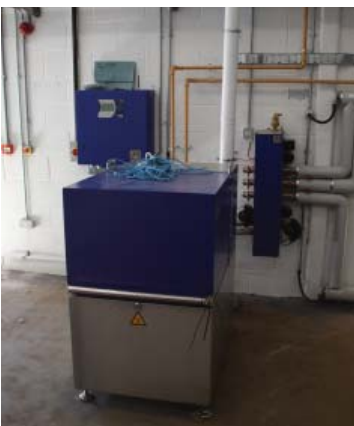
Plant room with Combined Heat and Power unit
