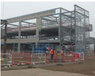
Steel frame construction on site: looking South through one of the colleges (top) and starting the weathertight boarding layer (bottom).
