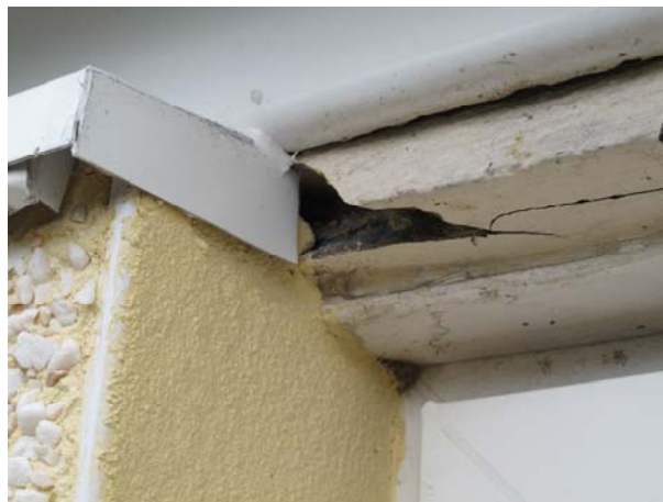
Figure 4.18 - Damage to window head during the installation of EWI
