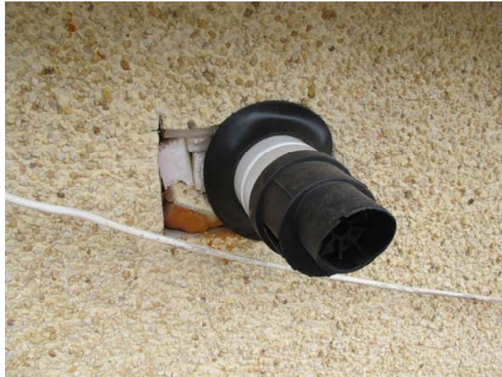
Figure 4.19 - Poor timetabling resulted in damaged EWI
