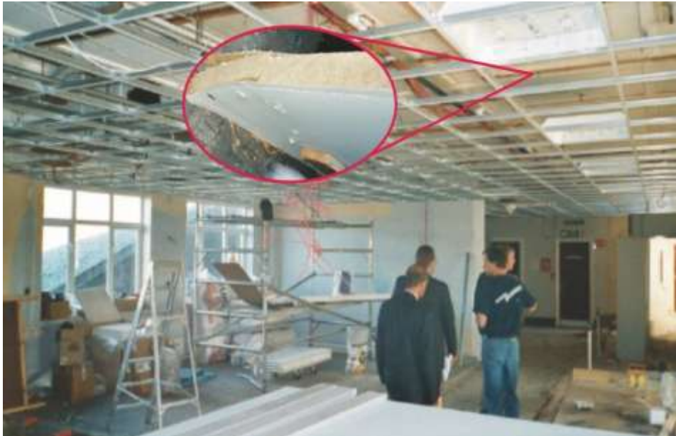
FIGURE 1: RENOVATION WORK INVOLVING THE STRAW BOARD CEILING (PHOTOGRAPH COURTESY OF DR R SMITH)
