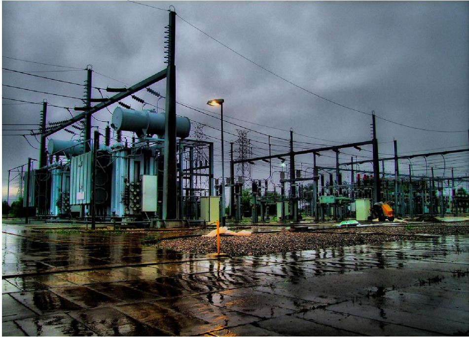
Figure 2.1: An example of an air insulated substation. Reproduced from [5].
