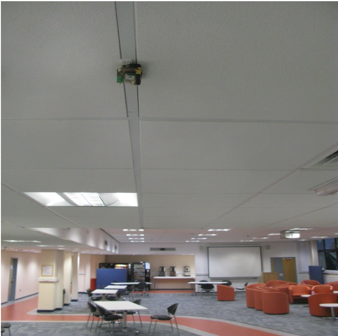
Figure 6.9 - A (typically) ceiling deployed ZigBee sensor host
