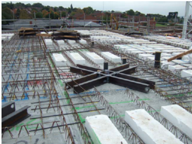
Figure 2. Two-way spanning filigree slab under construction by Laing O'Rourke plc at Stoke-on-Trent, UK, 2008
