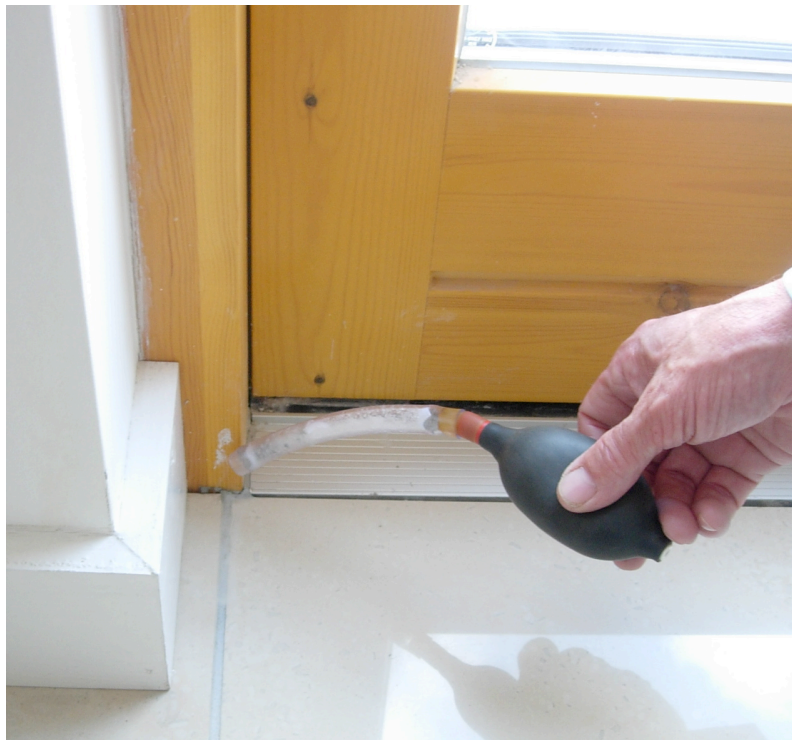
Figure 3: testing uncontrolled air leakage around a door frame using a smoke pencil. The strict control of air movement into and out of a dwelling represents a new experience for many builders and occupants, and is not always seen as a self-evident gain.
