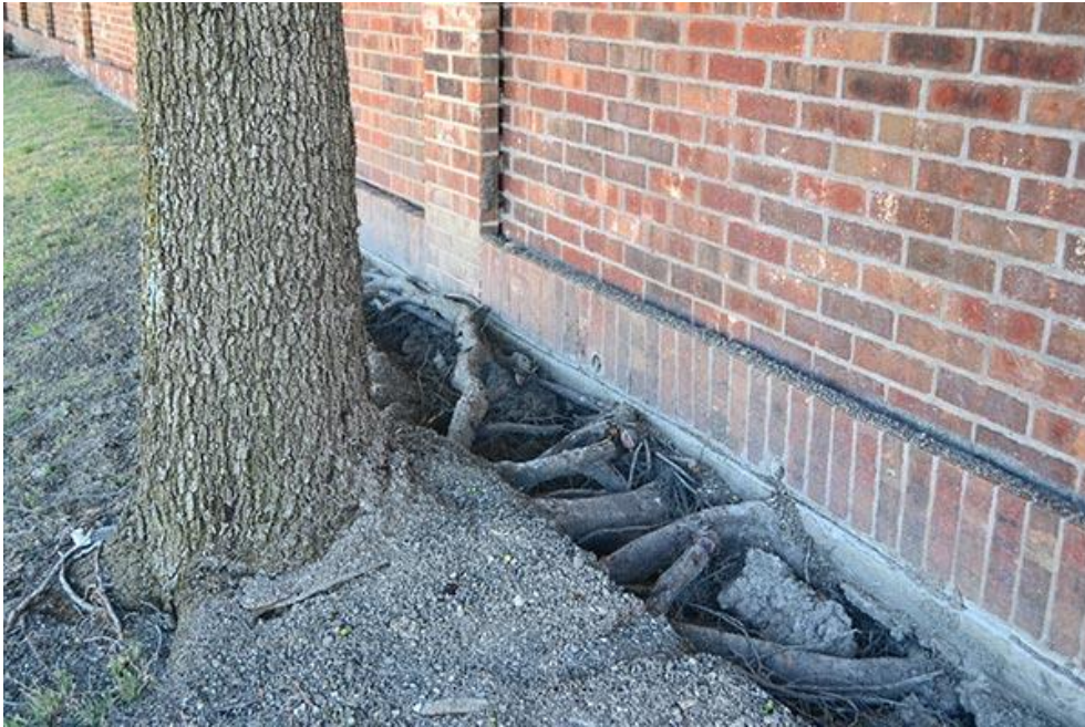
Figure 6: Tree roots growing under foundations (CNT Foundations, 2020)
