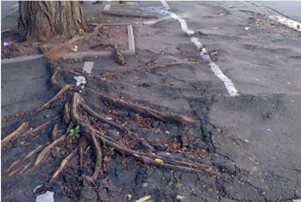
Figure 8: Damages to road pavement due to tree roots (Alani & Lantini, 2019)
