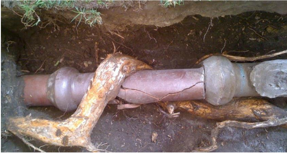
Figure 7: Roots growing around a pipe (911HVAC, 2019)
