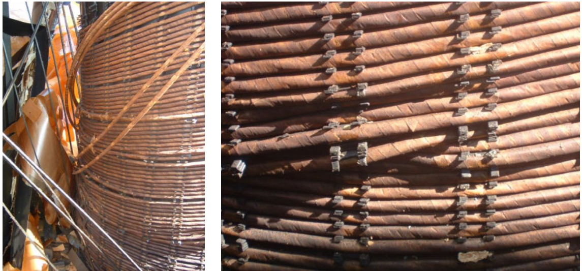
Figure 3-16 Winding Movement of Tap Winding from B Phase T2305
