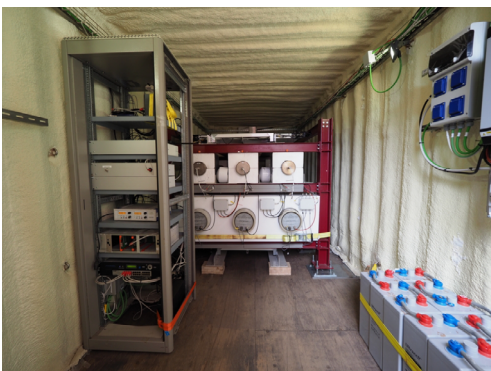
Figure 3: ORCA configuration into the maritime container.
