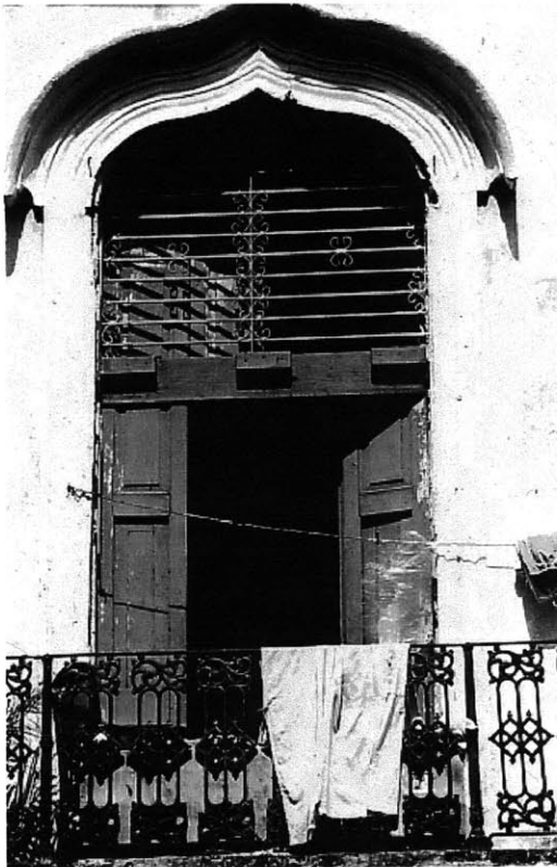
Typical view of a subdivided story. A barbacoa has been inserted. Bedroom space top level.
