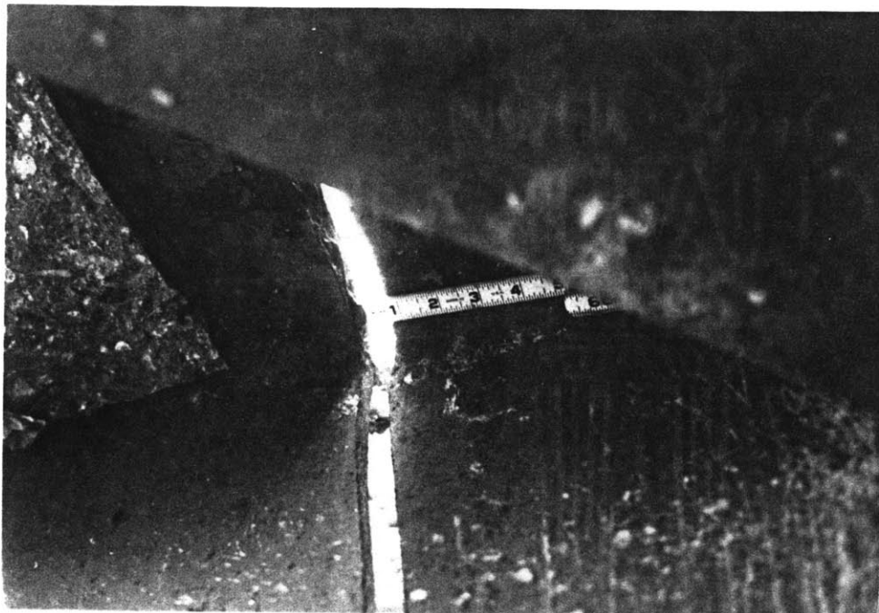
Photograph 6.6 Interior view of crack at bottom flange
