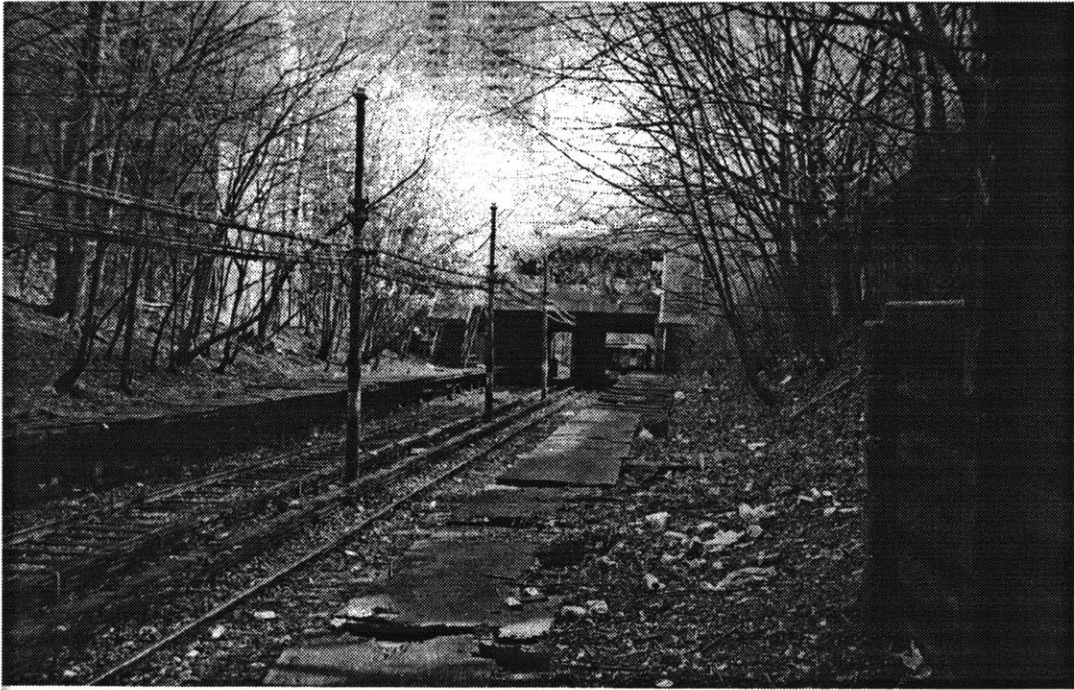
Photo #3: Botanic Garden Station Platform, April 1998. Looking Out on Closed Portion of Platform -- Deteriorated Wooden Planks
