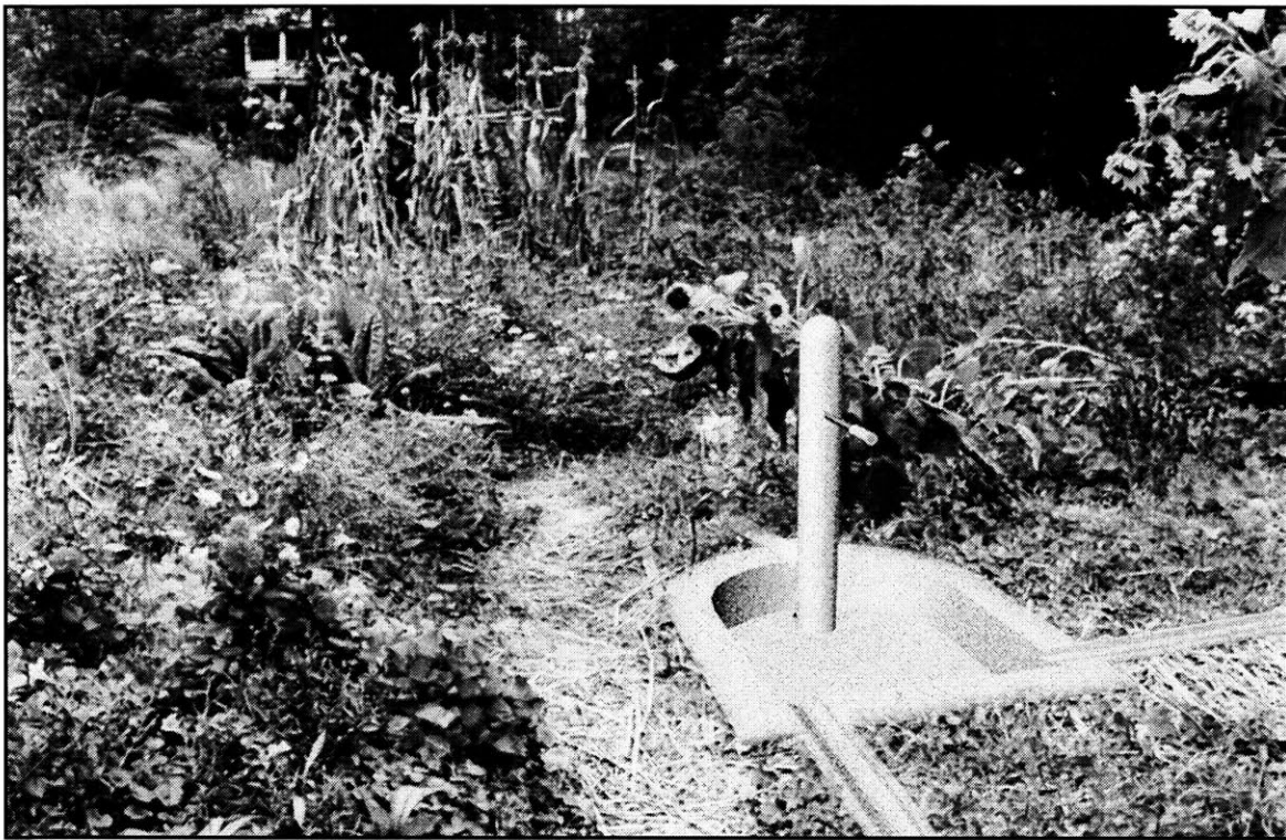
Pumping Station in the Garden- David B. Smith
