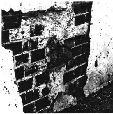
Figure 14: Typical deterioration of new construction
