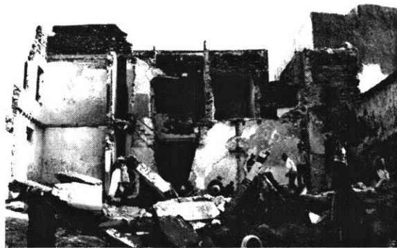
Figure 35: Collapsed house in the mellah, adjacent to ocean wall
