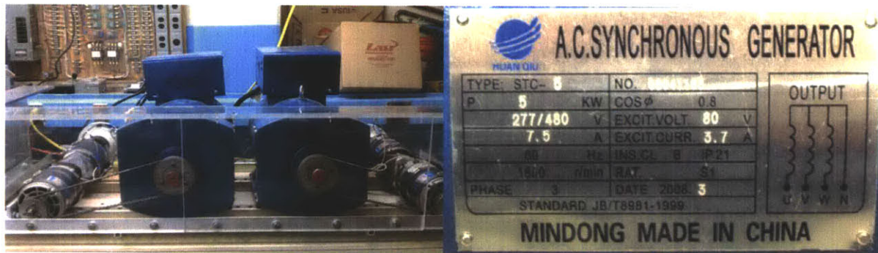
Figure 16: LEES Generator Setup and Specifications
