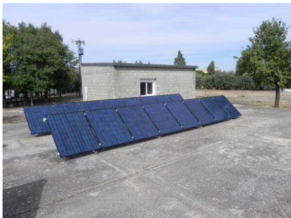
Figure 4. Photovoltaic field and building.
