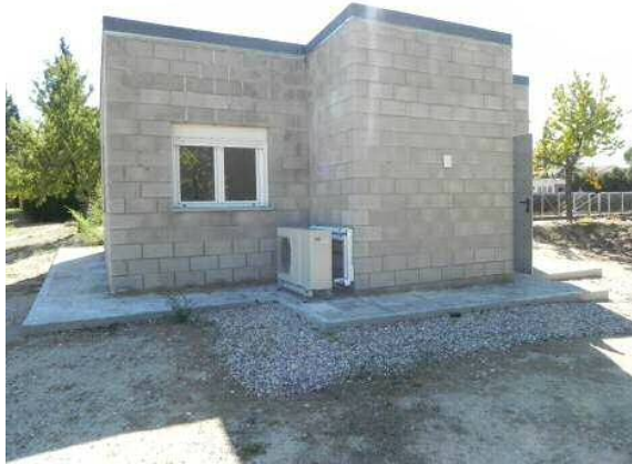
Figure 6. Air-water heat pump.
