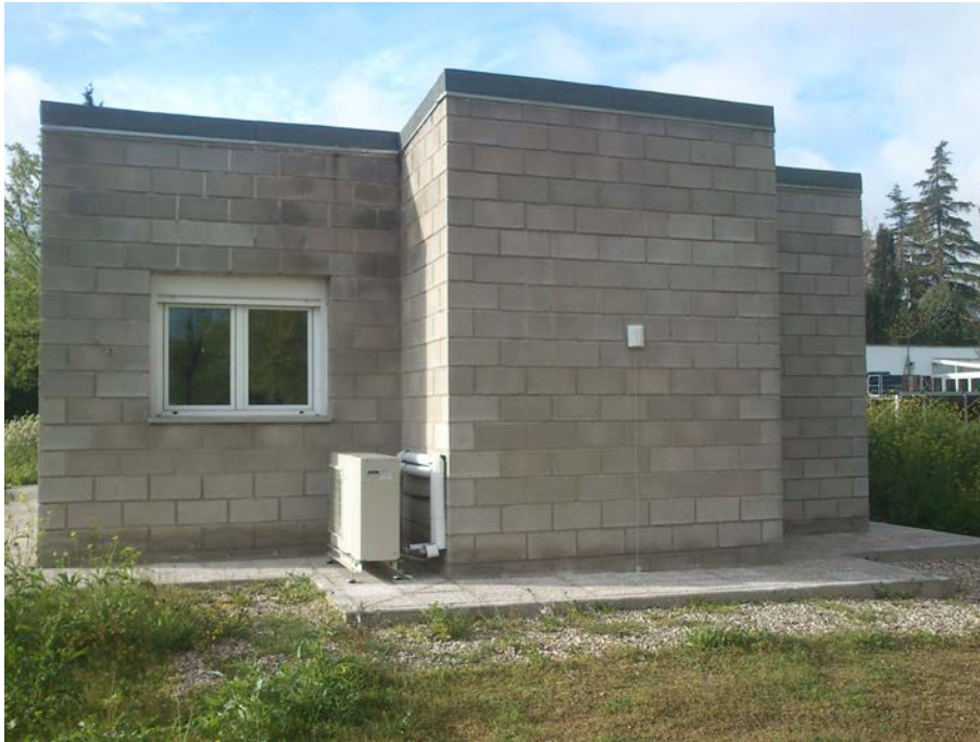
Figure 4.10: The heat pump out of the building.
