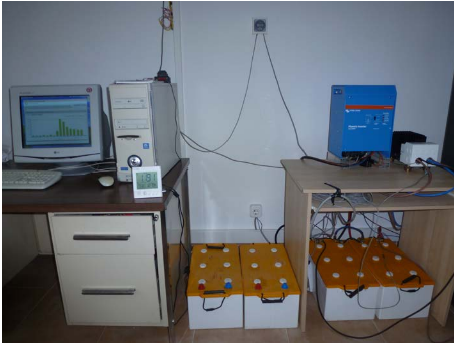
Figure 4.4: MPPT controller, inverter, storage system and registering equipment.
