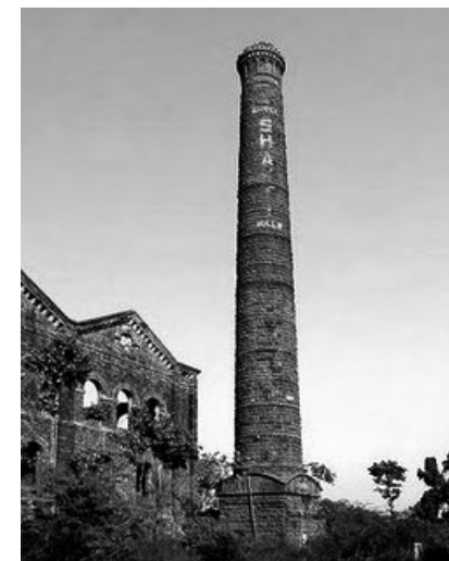
Chimney Stack to be conserved. NTC Mill Image Courtesy: Outlook Magazine ISLANDS
