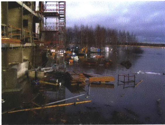
Construction in Arabiaranta, during a flood event. Image courtesy of Simo Haanpää.
