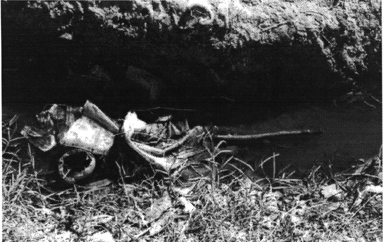
This clogged ditch is the wastewater collection and conveyance system for one unsewered area in La Plata.
