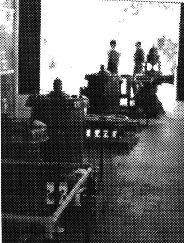
Pump motors at the Bosque Sewage Pumping Station
