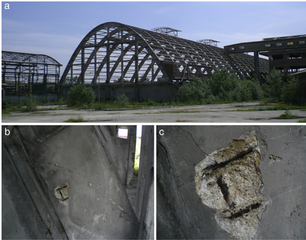
Fig. 1. a) Ex-Agrimont industrial plant, C3 building; b, c) concrete degradation on an arch in the south-western section of the structure.
