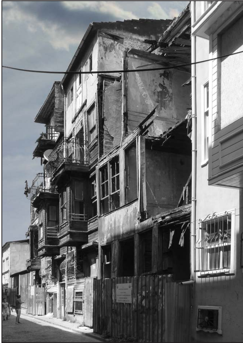
Figure 33: Partially collapsed buildings.
