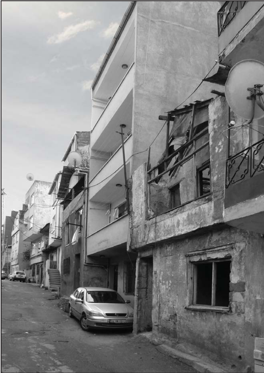
Figure 43: Partially collapsed structure.
