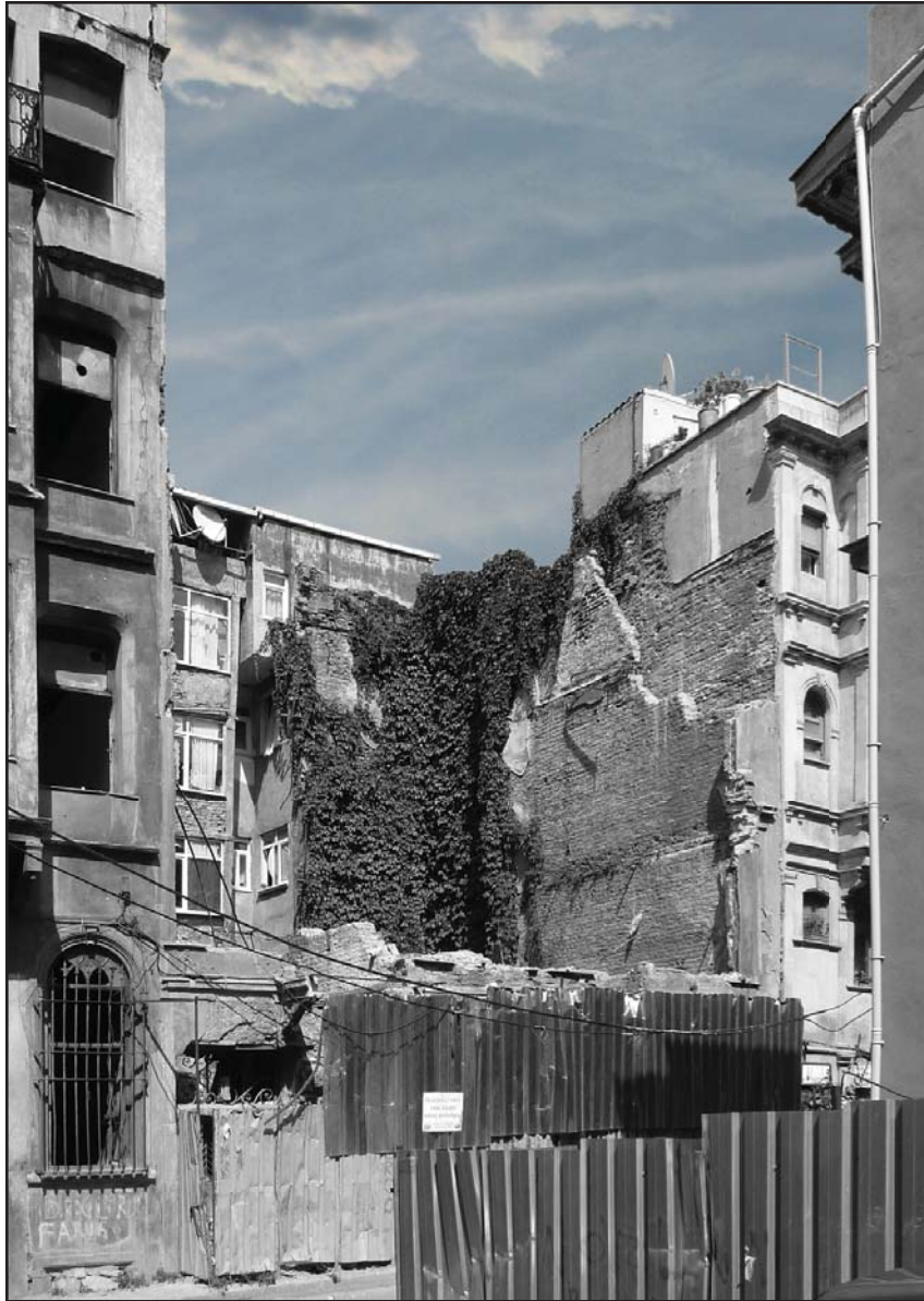
Figure 35: Collapsed and condemned buildings.
