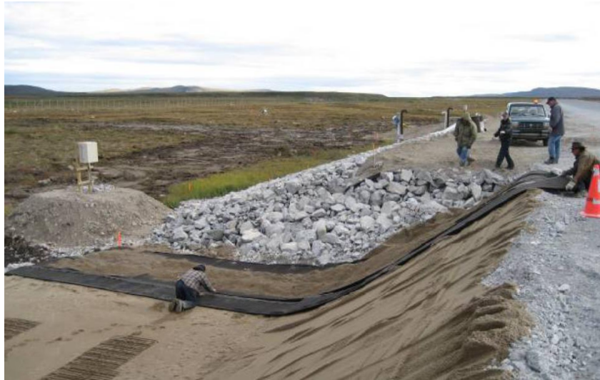
Figure 1. 13: Installing heat drain in the shoulder of Tasiujaq airstrip, Northern Quebec, Canada.
