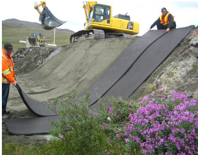
Figure 1. 14: Installing heat drain in the shoulder of the embankment at Salluit, Northern Quebec, Canada.
