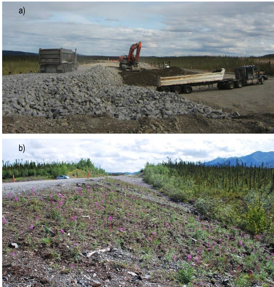
Figure A. 4: Full air convection embankment (S1) a) during construction; b) after construction.
