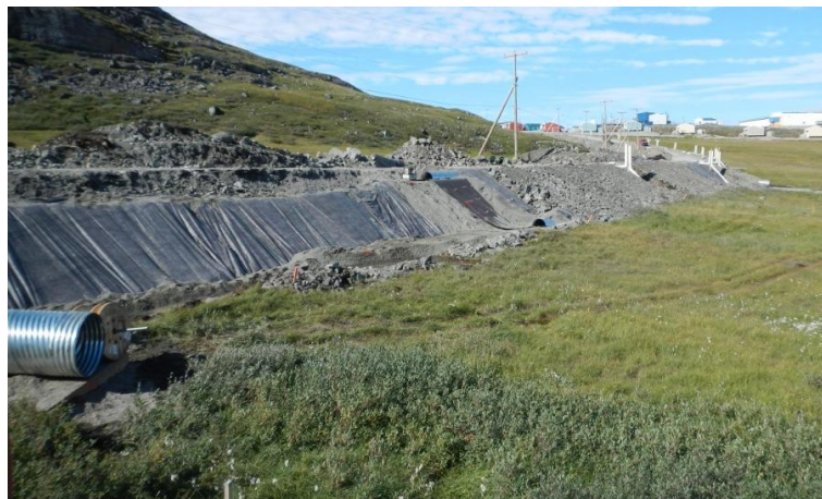
Figure 6. 12: The view of the roadway with heat drain installed in the shoulder at Salluit, Northern Quebec, Canada, providing the validation data.
