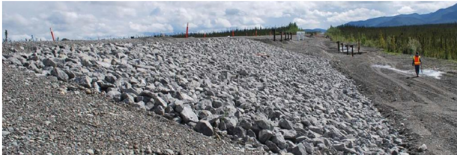
Figure A. 12: Air convection embankment on side slopes uncovered (S9) after construction.
