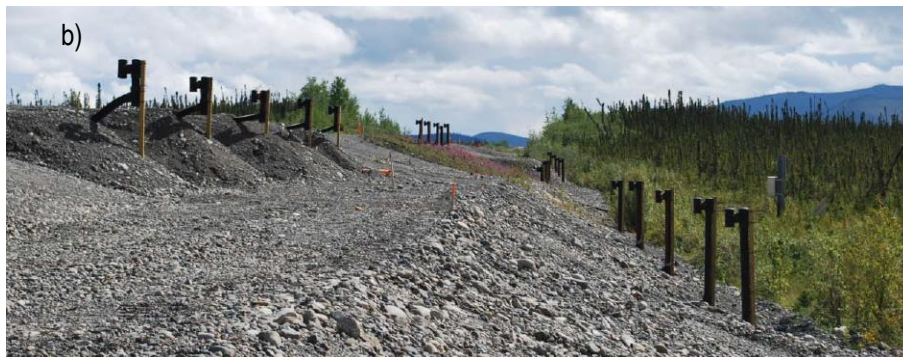
Figure A. 7: Heat drain in the side slope (S4) a) during the construction; b) after the construction.
