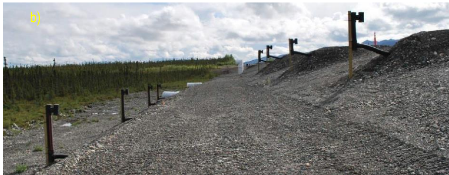
Figure A. 11: Heat drain in side slopes with insulation (S8) a) during construction; b) after construction.
