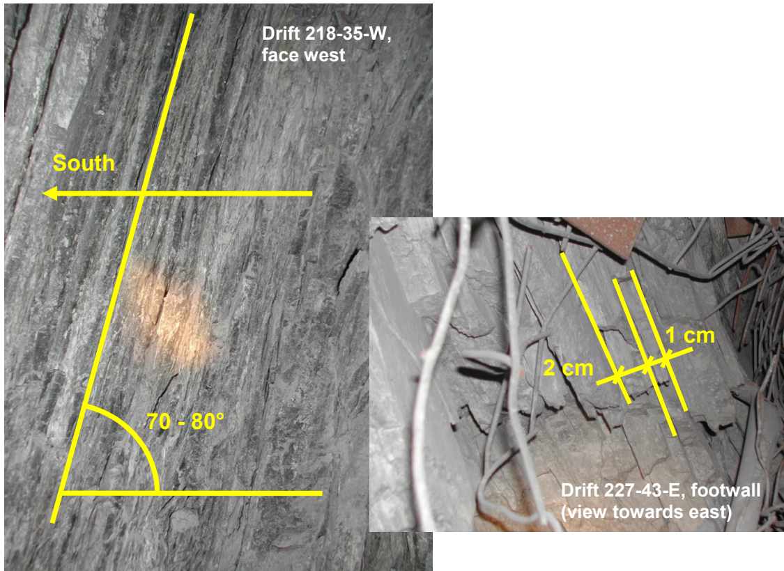
Figure 54: Foliation of rock (tuff) in drift 218-35-W and 227-43-E at the LaRonde mine
