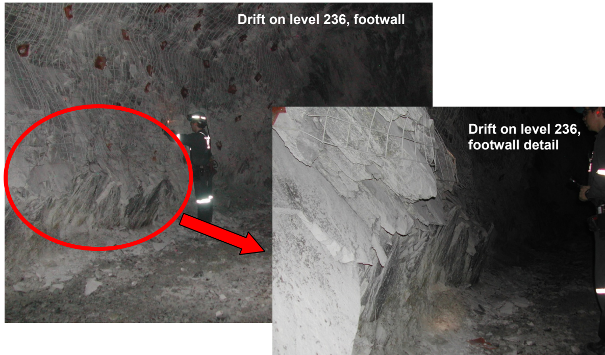
Figure 45: Drift wall deformation due to squeezing, observed at LaRonde on level 236 (Feb. 2008)
