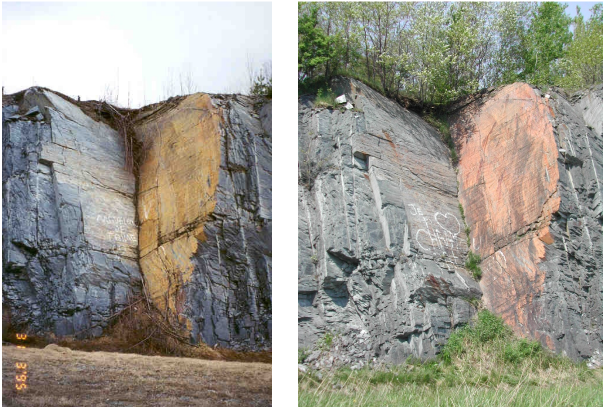
Figure 13: Sliding planes of a wedge failure (wedge B) observed at the Fleurimont rock slope: March 31, 1995 (left) and May 24, 2007 (right)
