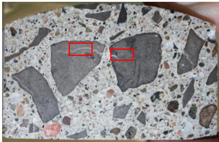
Figure 6.3 Picture of the concrete surface with an indication of the zones for micro-indentation testing (rectangular windows).
