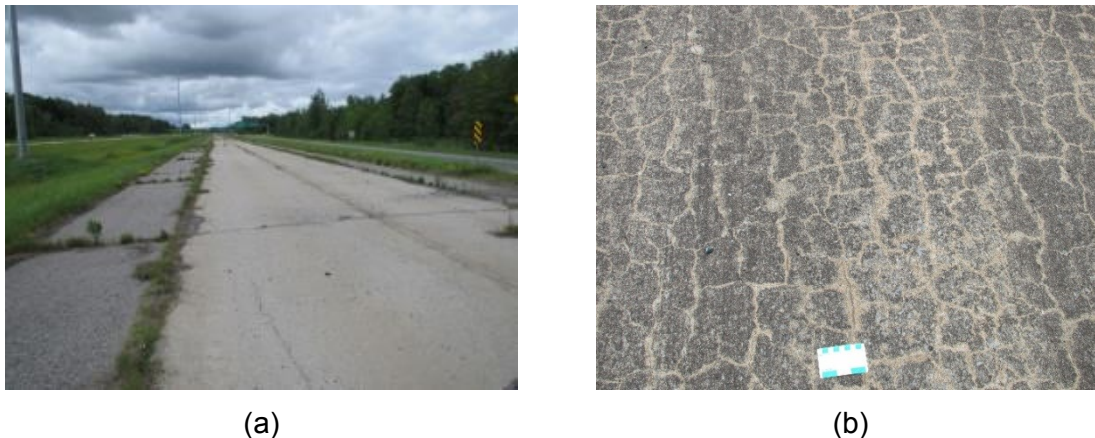
Figure 4.1 (a) General view of the Becancour concrete pavement; (b) Surficial condition of the pavement section from which the cores used for the testing program were extracted.
