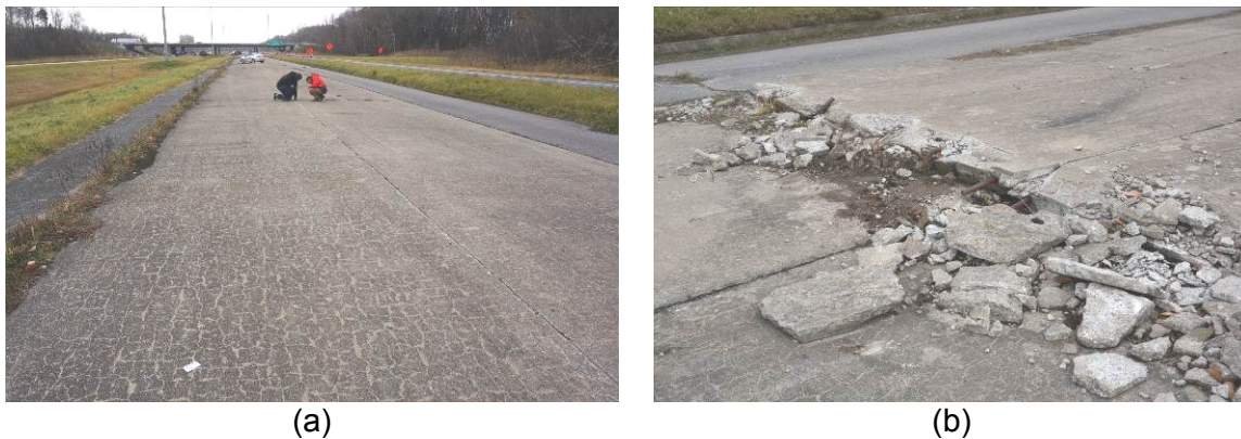
Figure 6.2 (a) The pavement in Trois-Rivières made with reactive Trenton limestone and showing extensive map cracking; (b) Bursting at a joint of the pavement.
