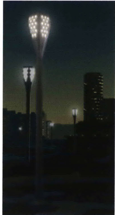
Fig. 3.3. Philips LED luminaire which responds to different ambient light conditions.
