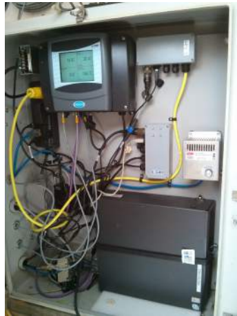
(a) Installed equipment inside the Primodal RSM30.
