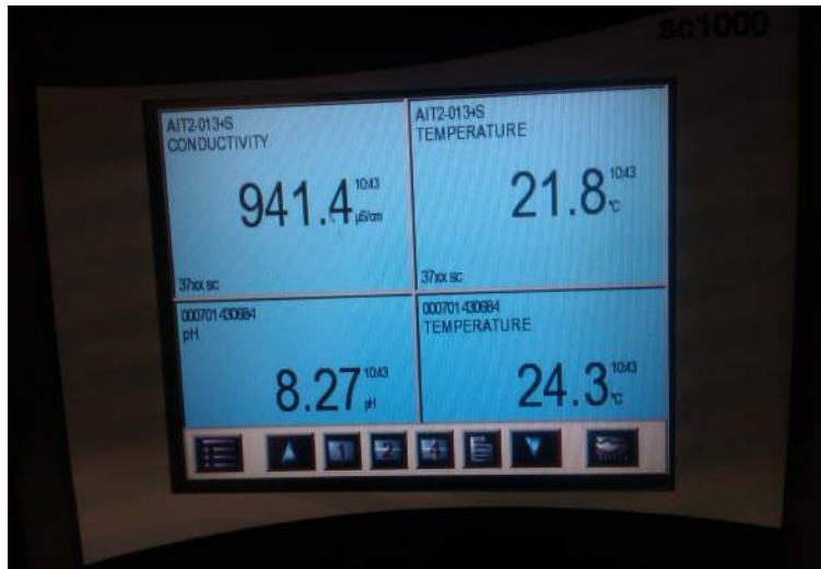
Figure 3.22: Interface and color touch-screen display of the sc1000 controller (Hach, 2012).
