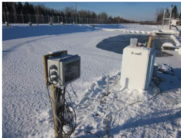
Figure 4.13: Protection for the cable connections at the Wemotaci F/AL.
