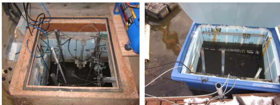
(a) Sensors support at the inlet of the Wemotaci lagoon. (b) Sensors support at the outlet of the Wemotaci lagoon.
