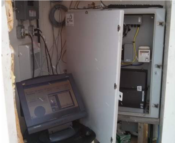
Figure 3.8: Installed Primodal RSM30 cabin.
