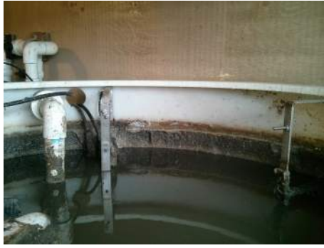
(a) Sensors support at the inlet of the Grandes-Piles F/AL.
