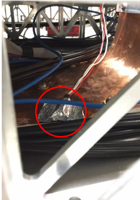
Figure 60: Thermocouple placement for the 128 Controller strap
