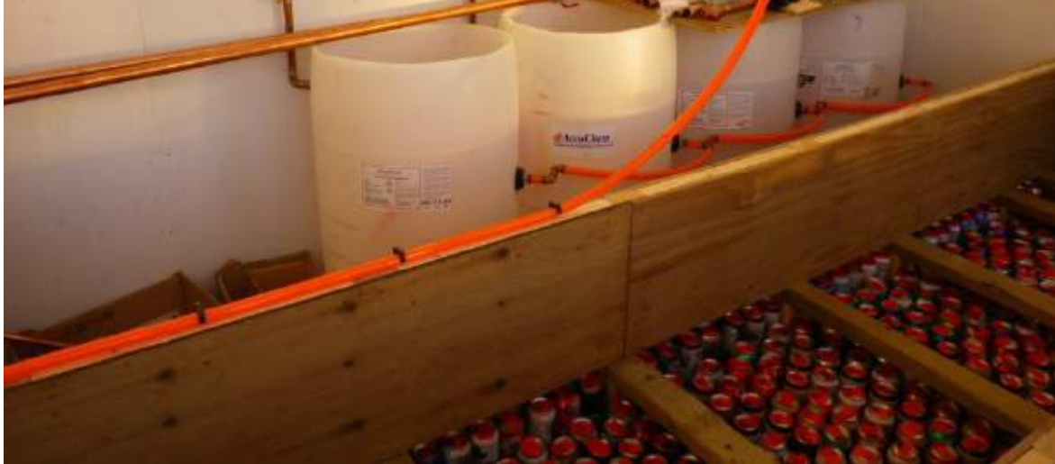
FIGURE 19 Thermal storage and heat modulation system, Yukon College Greenhouse.
