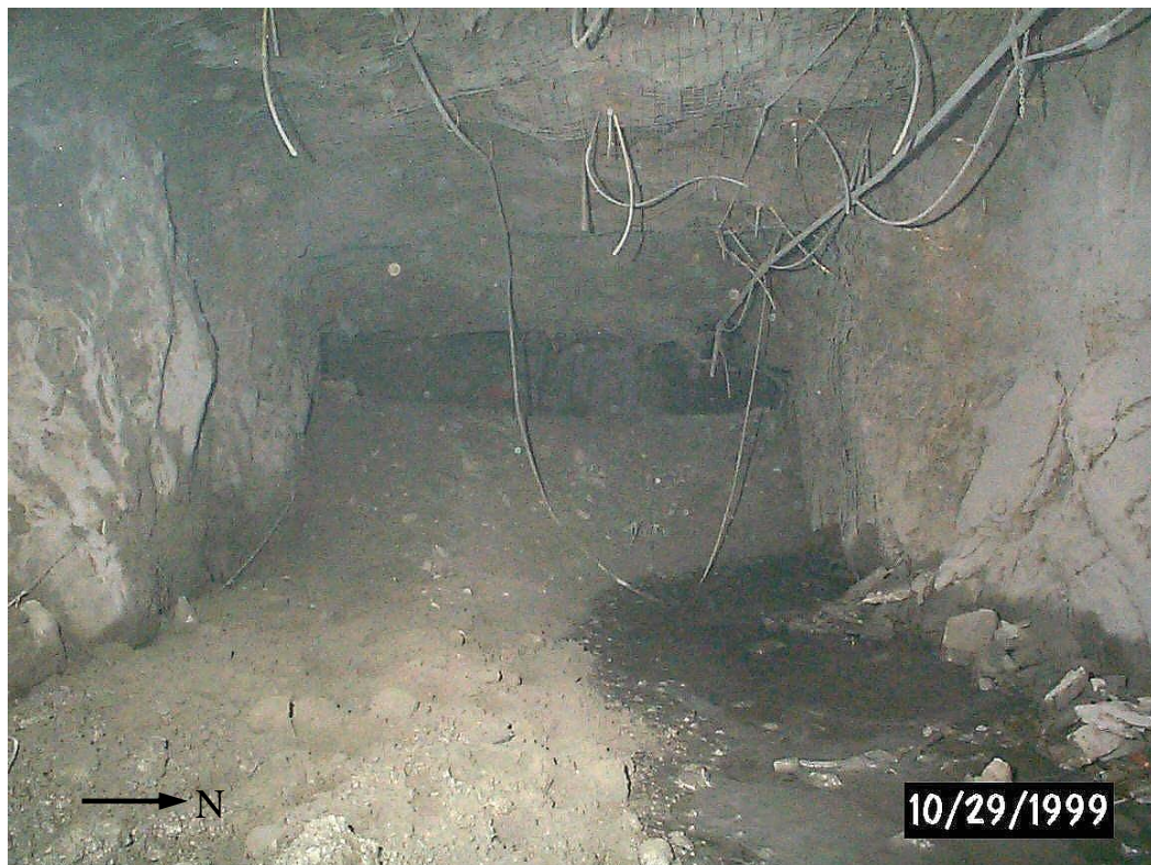
Figure 67. Photograph looking west taken on 1000 Sill in the access cross-cut to the 29-9 Pillar. (After Andrieux et al. , 2000.)
