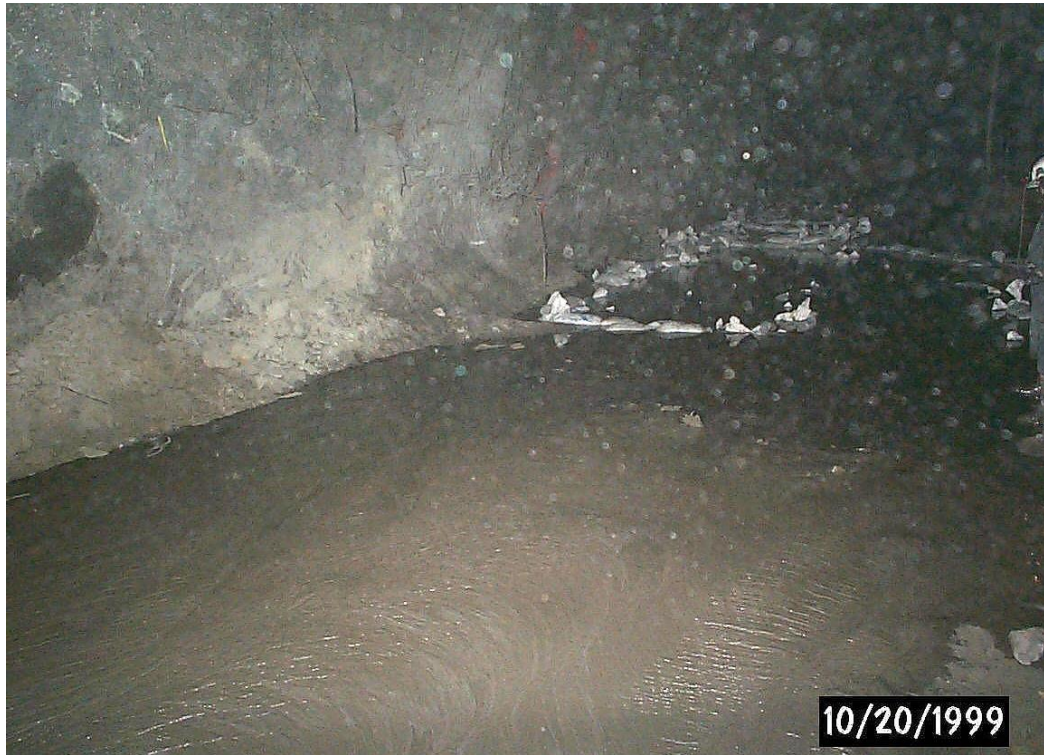
Figure 61. Photograph looking northwest from the pillar access showing the placement of the 7% cement paste backfill. (After Andrieux et al. , 2000.)
