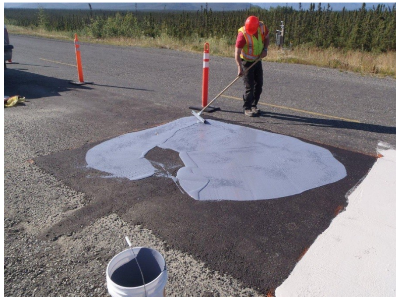
Figure 3.3: Installation de l'enduit Perfect Cool A de Nippo (Photo: Yukon Highways and Public Works)
