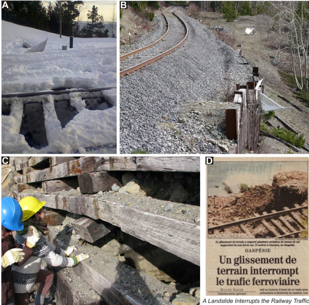
Figure 4-7 Examples of damage caused by the accumulation of displacements on the infrastructures and of the 1998 collapse event. A) Undermining of the railway ballast in an underlying fissure in February 2011. B) Deformation of the retaining wall and of the railway. C) Deformation in the retaining wall built in 1998 D) Newspaper cut showing the damaged railroad after the 1998 slide event (Le Soleil, 1998).
