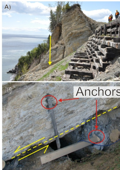
Figure 9. A) Position of the crackmeter F12 and looking west at the Petit-massif B) F12 is installed to monitor a translational movement of the upper block relative to the lower block. F11 is measuring the opening of the crack below F12.
