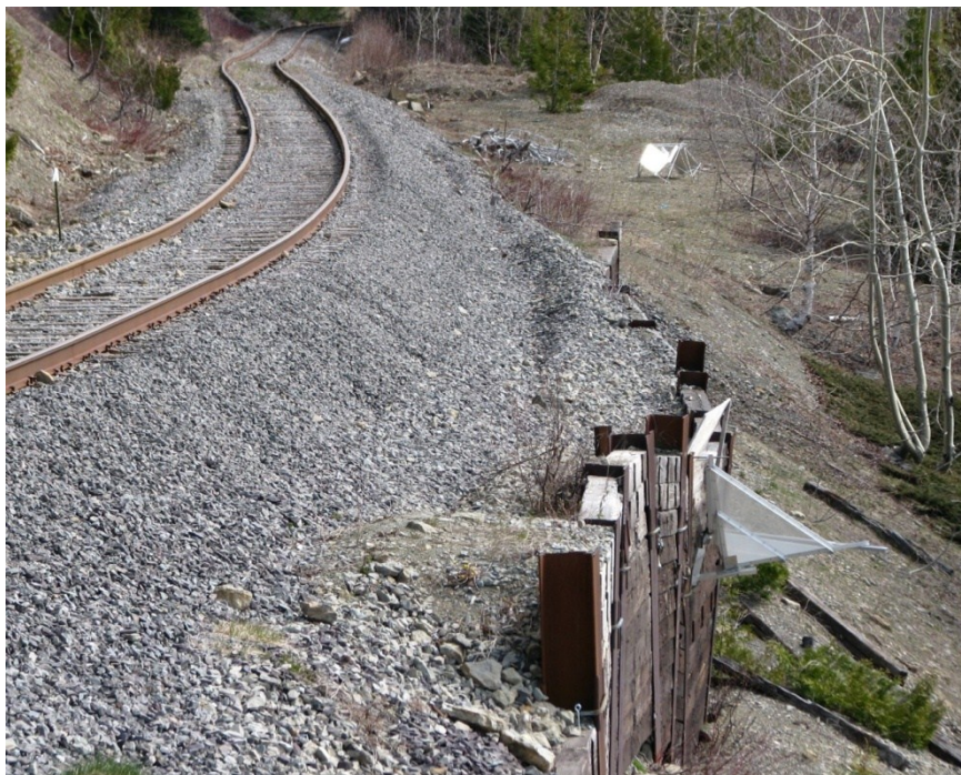
Figure 3-5 View towards the east showing deformation of the railroad with a clear departure from a straight line at the eastern limit of the rockslide. The horizontal displacement from the initial alignment is estimated to be about 1 m from the observation of aerial photographs and DEM.
